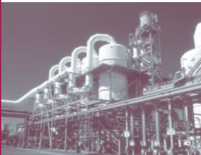
Western Mining Corporation's sulphuric acid plant.
